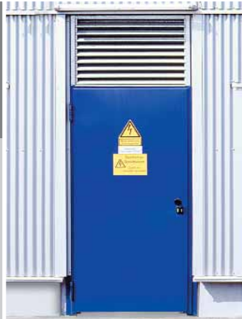
Transformer doors Ventilation louvres
